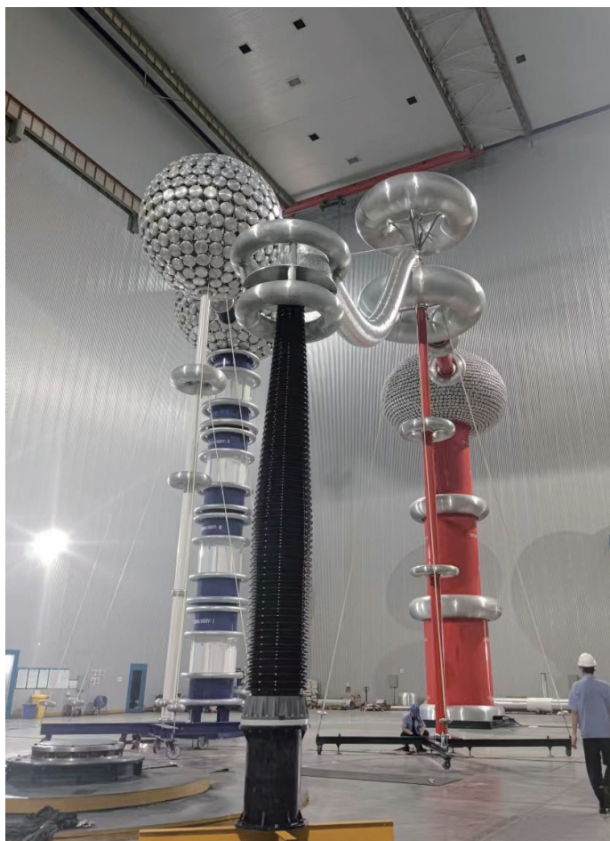
◎ SF6 气体绝缘套管 (瓷) SF6 gas-insulated bushing (Porcelain)
